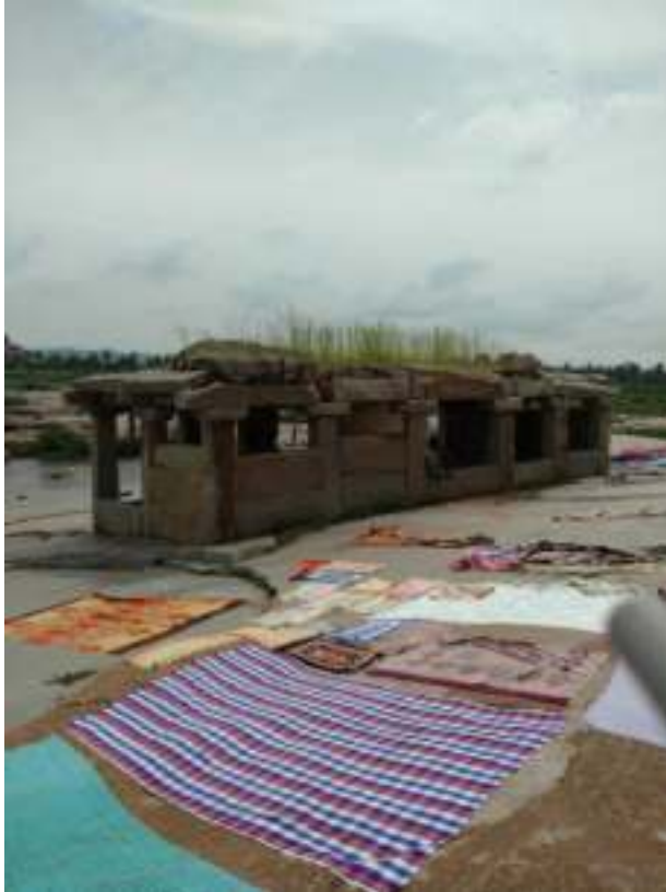
Figure 1: Roof of 1st Mantapa needs be restored.
