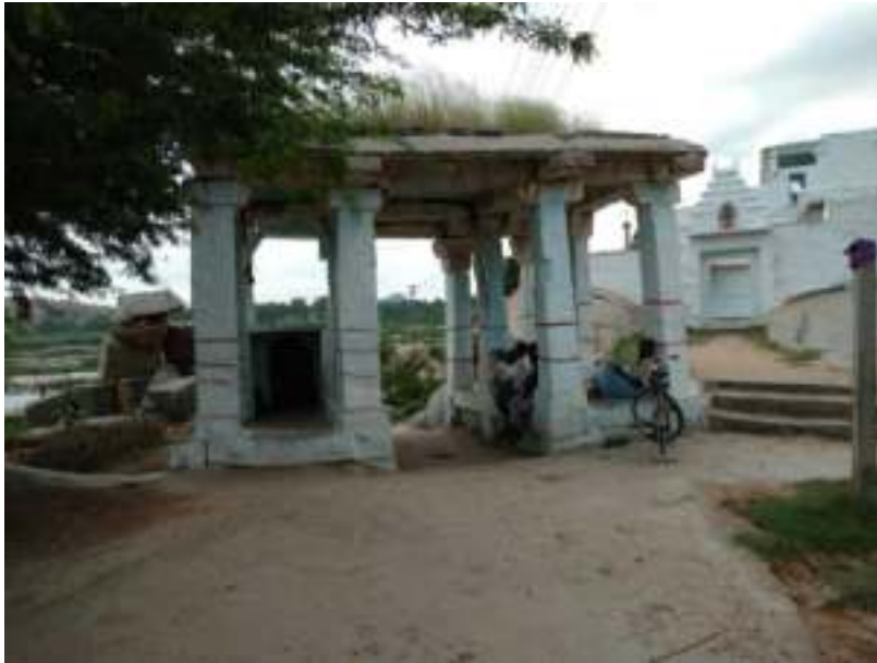
Figure 3: 2 nd Mantapa, the roof needs to be restored.
