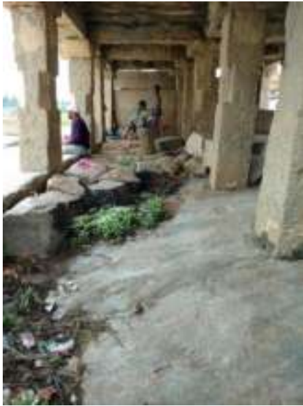
Figure 6: The interiors of the Mantapa need to be cleared and the flooring needs to be raised using flagstones/lime slurry.
