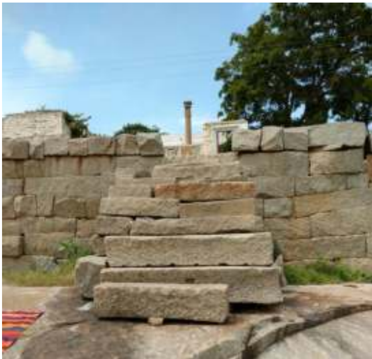
Figure 11: Steps of the fort wall need to be restored.
