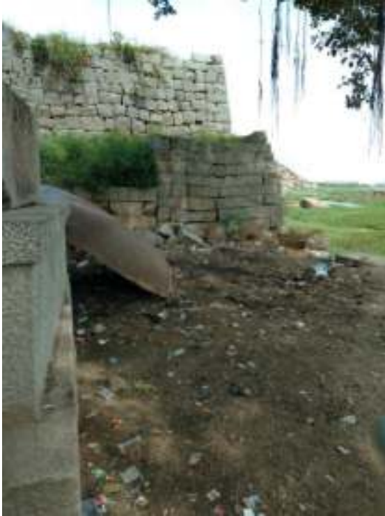
Figure 14: At the Snanaghatta area - garbage needs to be cleared, the earth should be levelled.
