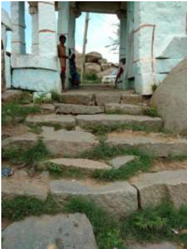
Figure 7: Present condition of the steps. The approach needs to be reconstructed.
