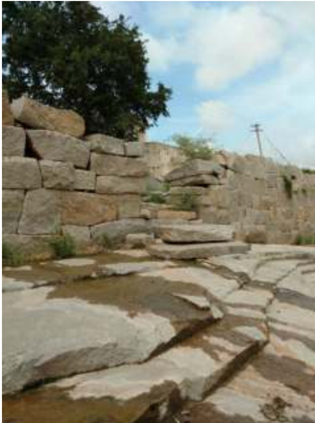
Figure 12: Steps need to be reinstalled.
