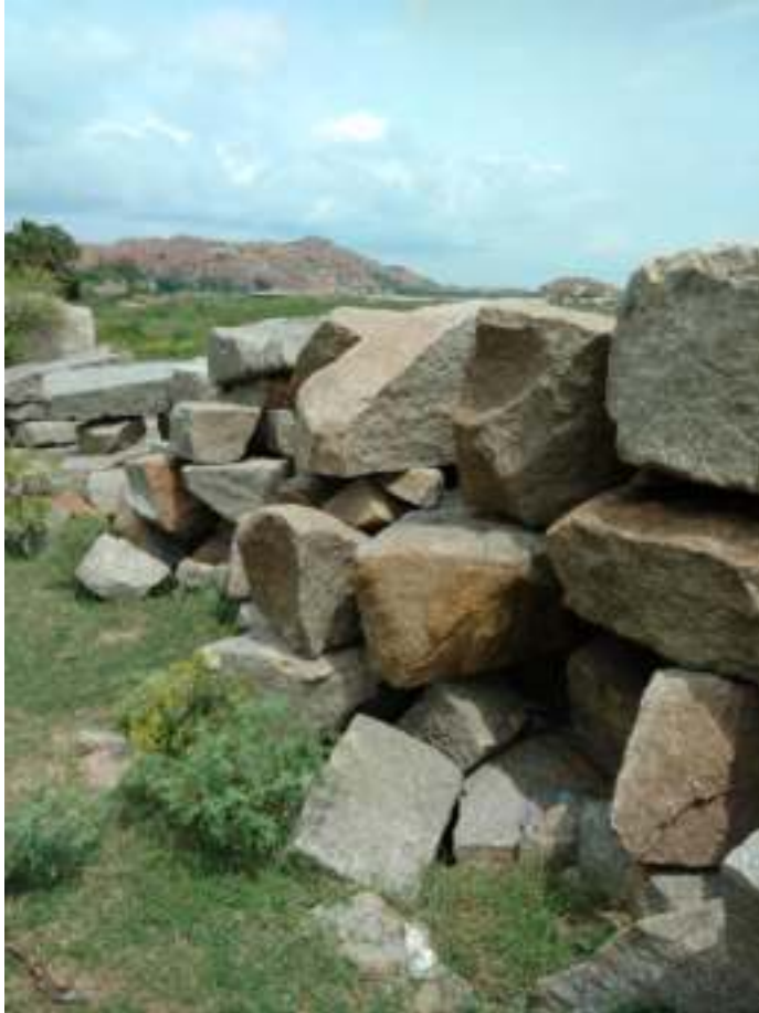
Figure 10: The inner facade of the fort wall requires complete reconstruction with ancient stones.
