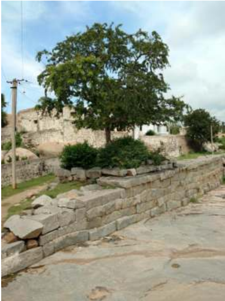
Figure 9: River front facade of the fort wall - the facade is in a good condition - minimal restoration required.
