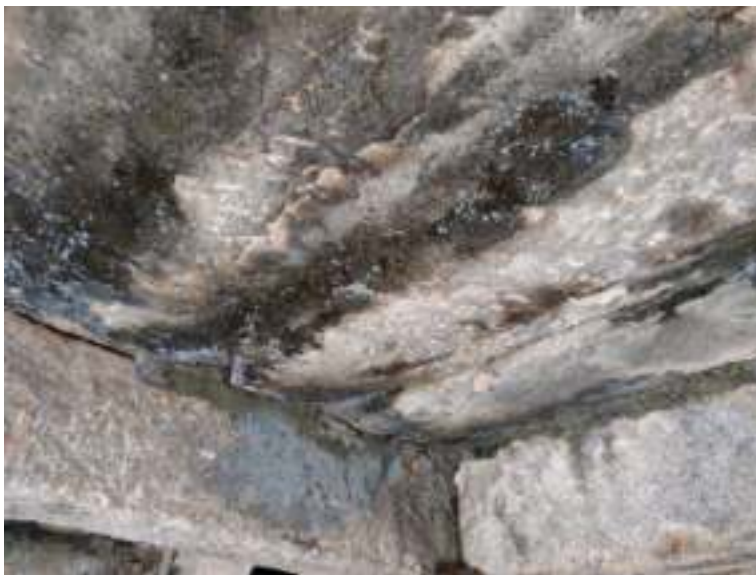
Figure 2: 1st Mantapa, water ingress is seen in the soffit of the roof.
